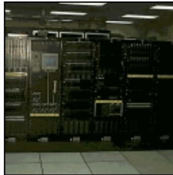
2.2.1.2.5c VCSS/EVTS Equipment Racks (BS-4)
