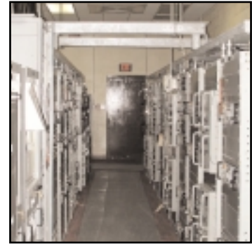
2.2.1.2.5b Equipment Room with Racks
