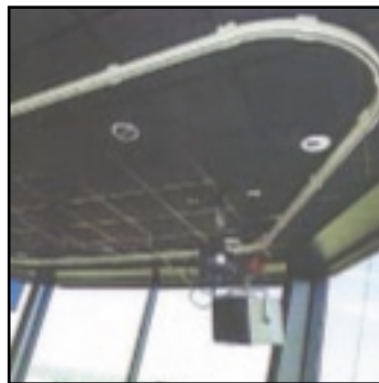
1.2.1.7.c Tower Radar Display Equipment
