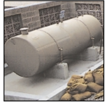
1.2.2.15 Typical Fuel Oil Storage Tank
