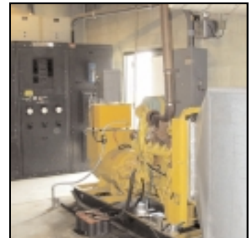
2.3.1.2.2.1 Generator in Generator Room
